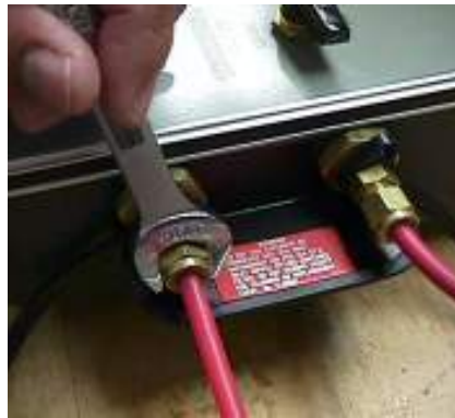
Connect instrument to be tested to the OUTLET valve.
